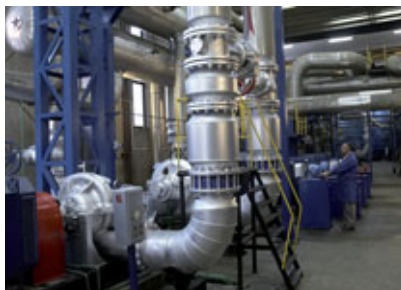
Heating and air-conditioning technology
